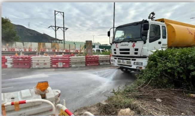
利用水車清洗工地附近的公路 Cleaning of adjacent public roads by water truck
