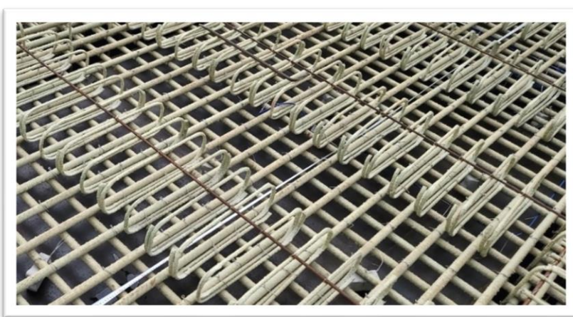
「重建南丫島北角碼頭工程」混凝土層板結構的玻璃纖維筋 GFRP rebars in concrete slab under the reconstruction of Pak Kok Pier on Lamma Island
