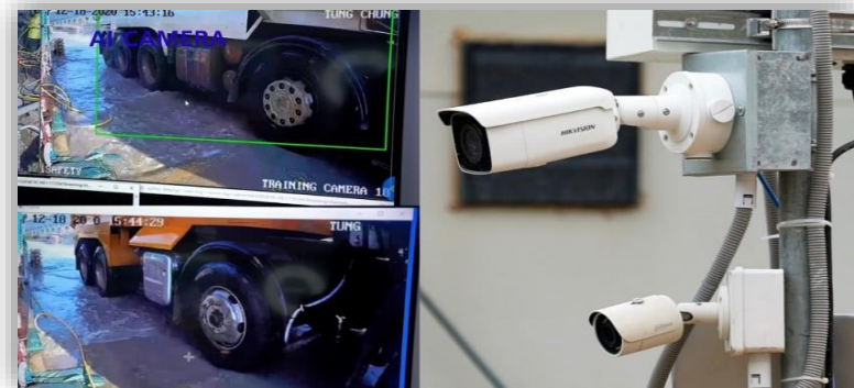
人工智能攝像鏡頭監控自動洗車池 Automatic wheel washing system monitored by AI camera
