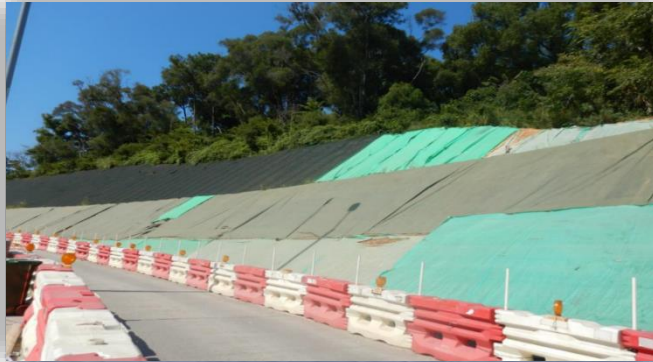
用防水布覆蓋斜坡防止揚塵 Covering of fill slope to prevent dust dispersion
