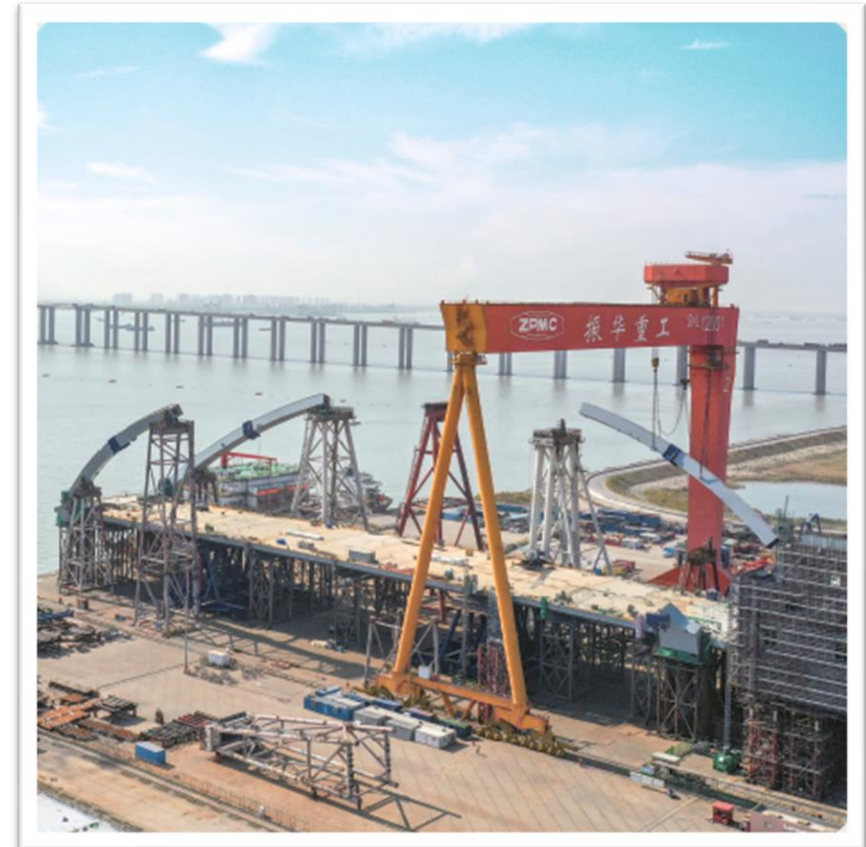
於國內工廠預製鋼拱橋 Prefabrication of steel arch bridge at Mainland yard
